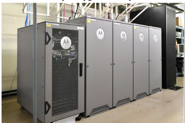
Figure 5 TETRA radio base station at Narita International Airport
