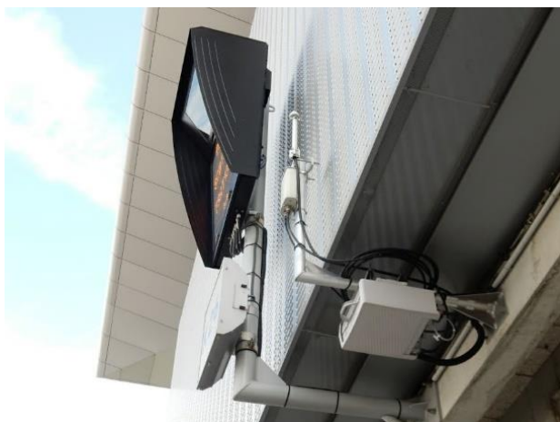
Figure 10 Private LTE base station in Charles de Gaulle Airport of Paris
